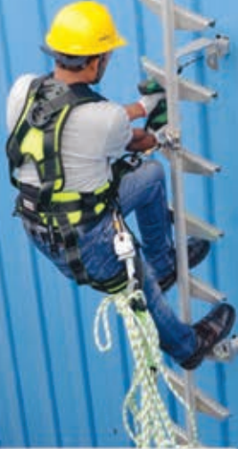
Vertical Ladder System
